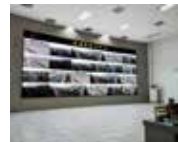
Expressway monitoring centre
